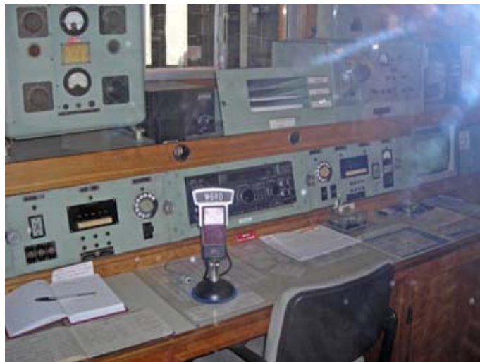
W6RO operating position. [Photos by W2CH]
